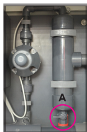
Reactor Leakage Device
